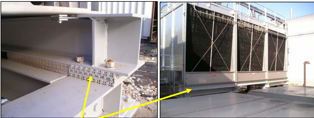
AirLoc B4 pads installed under the Marley cooling towers
